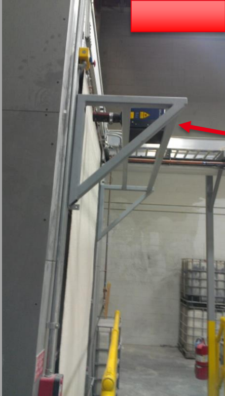
Exit of Oven
